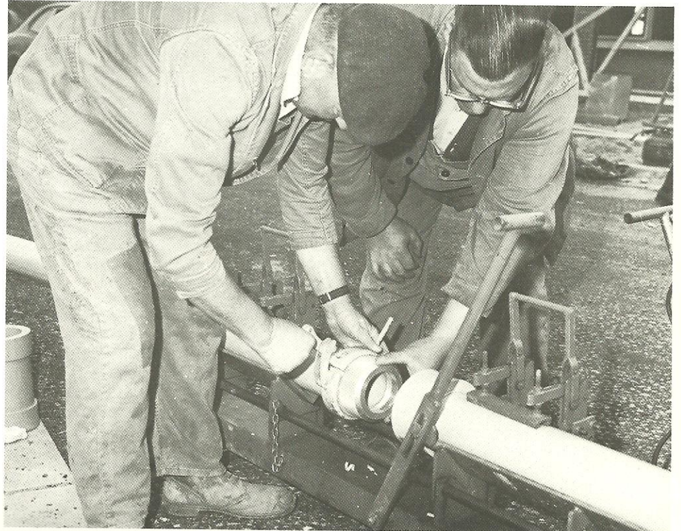
A depth gauge tool is used to measure the socket for the joint.
